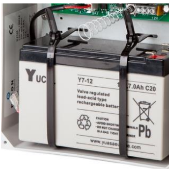
2 x Battery restraining ties
